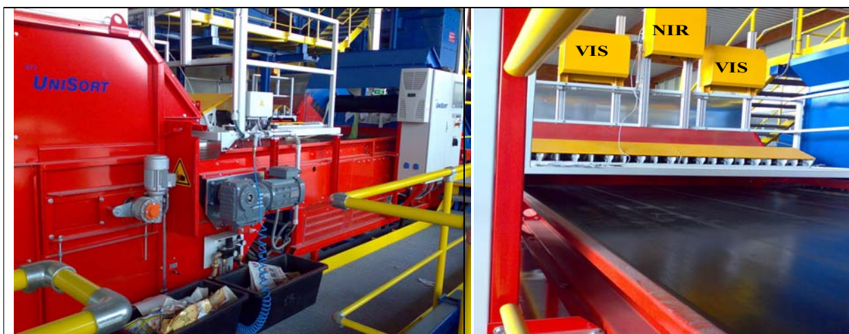
UNISORT Unit integrated into new sorting plant
